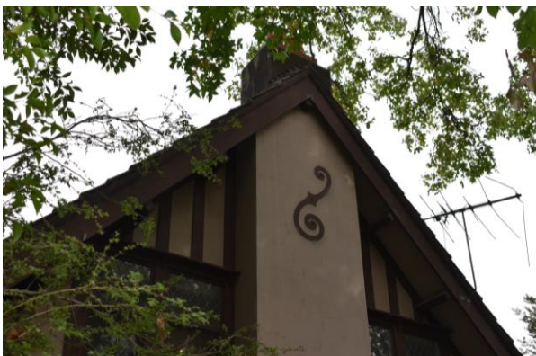
Detail view of S shaped wall tie and chimney breast (source: Extent Heritage Pty Ltd, 2022).
